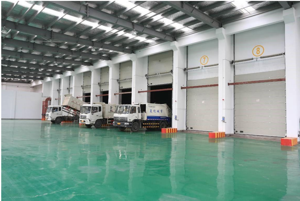
Figure 7: Waste receival hall showing trucks unloading into the waste bunker
