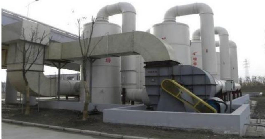
Figure 8: Image of the secondary odour control scrubber
