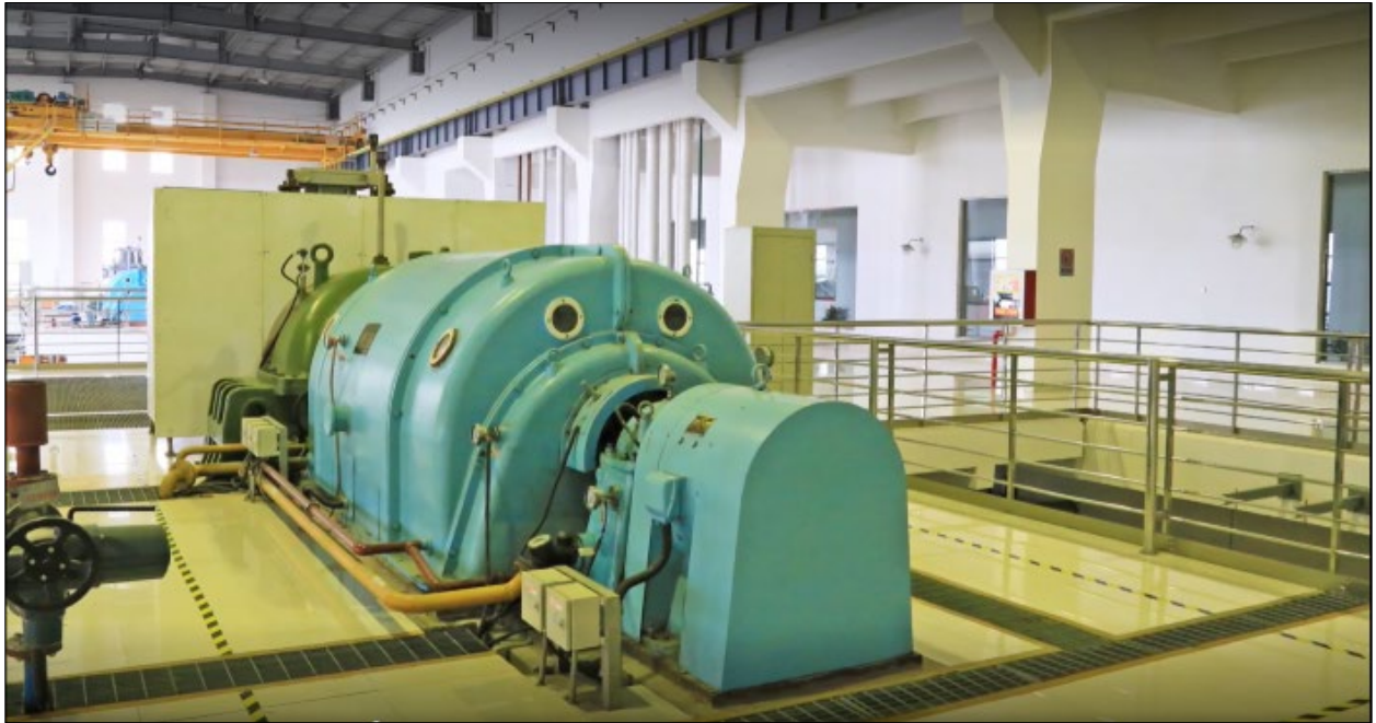
Figure 32: Steam turbine and generator
