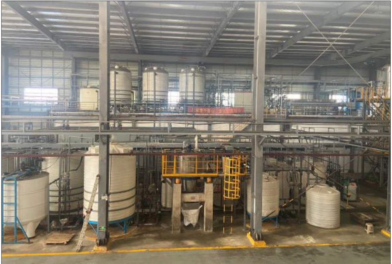
Figure 26: Plasma wastewater treatment plant
