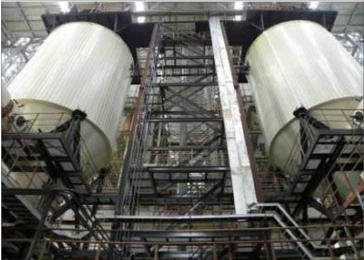
Figure 19: Dual semi-dry deacidification reaction towers
