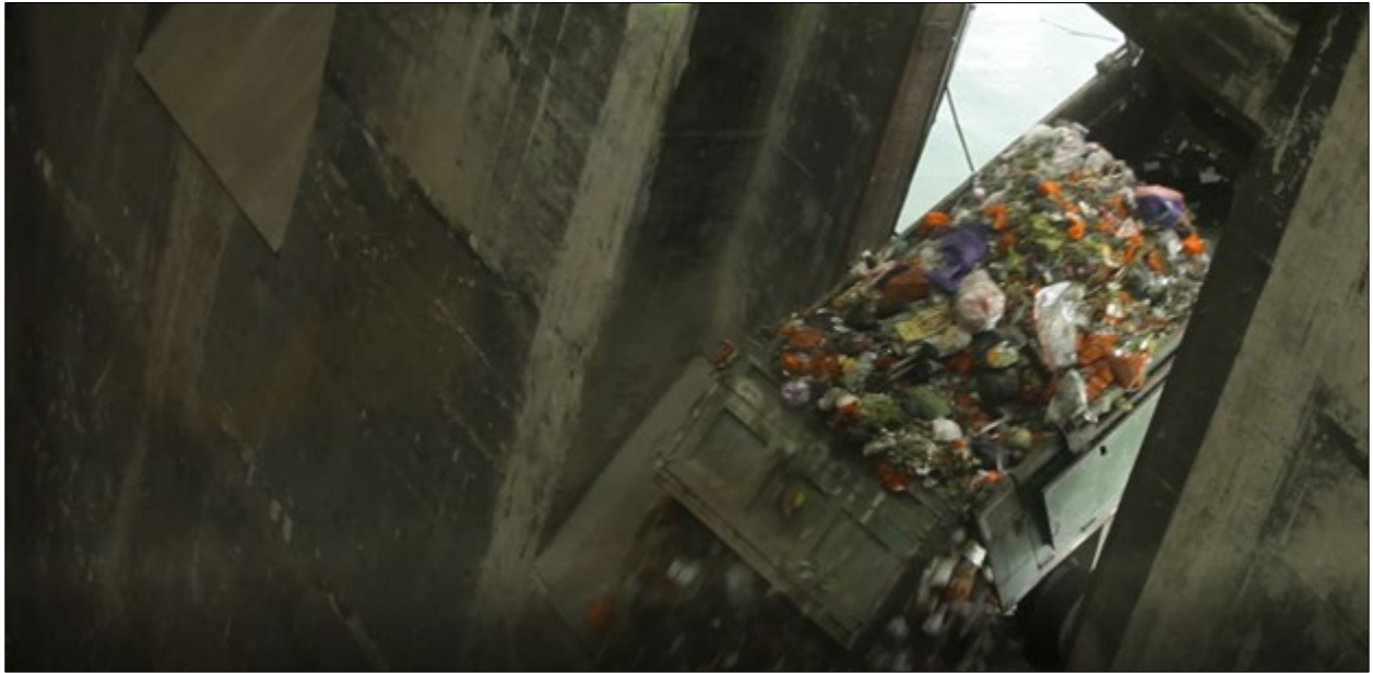
Figure 8: Truck tipping waste from the unloading floor into the waste bunker
