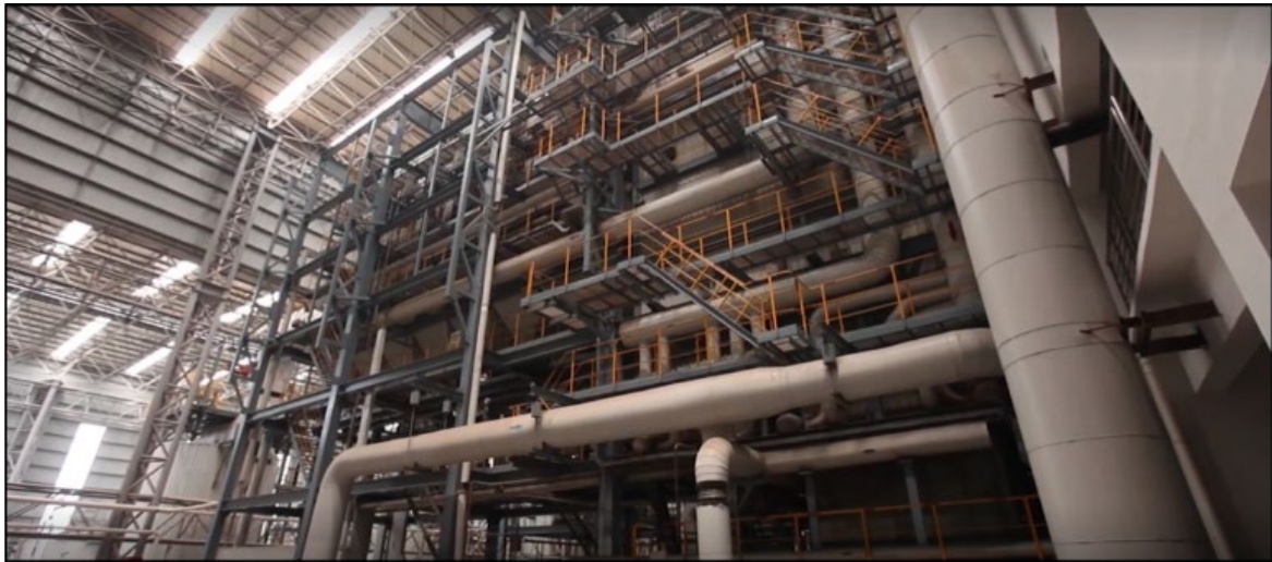
Figure 14: Boiler and heat recovery system
