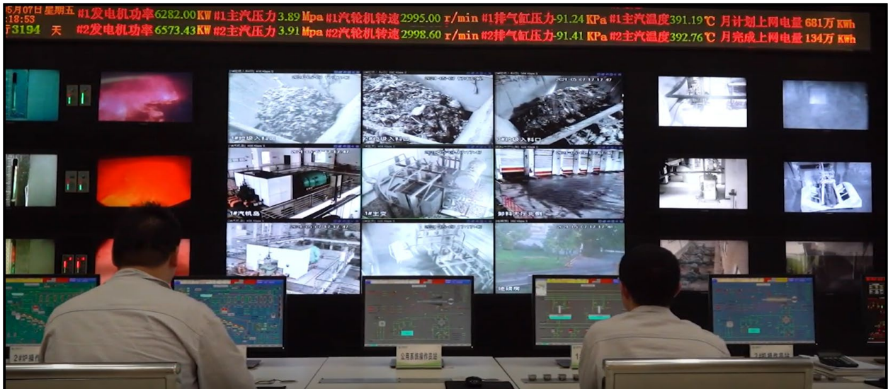
Figure 27: Main process control room
