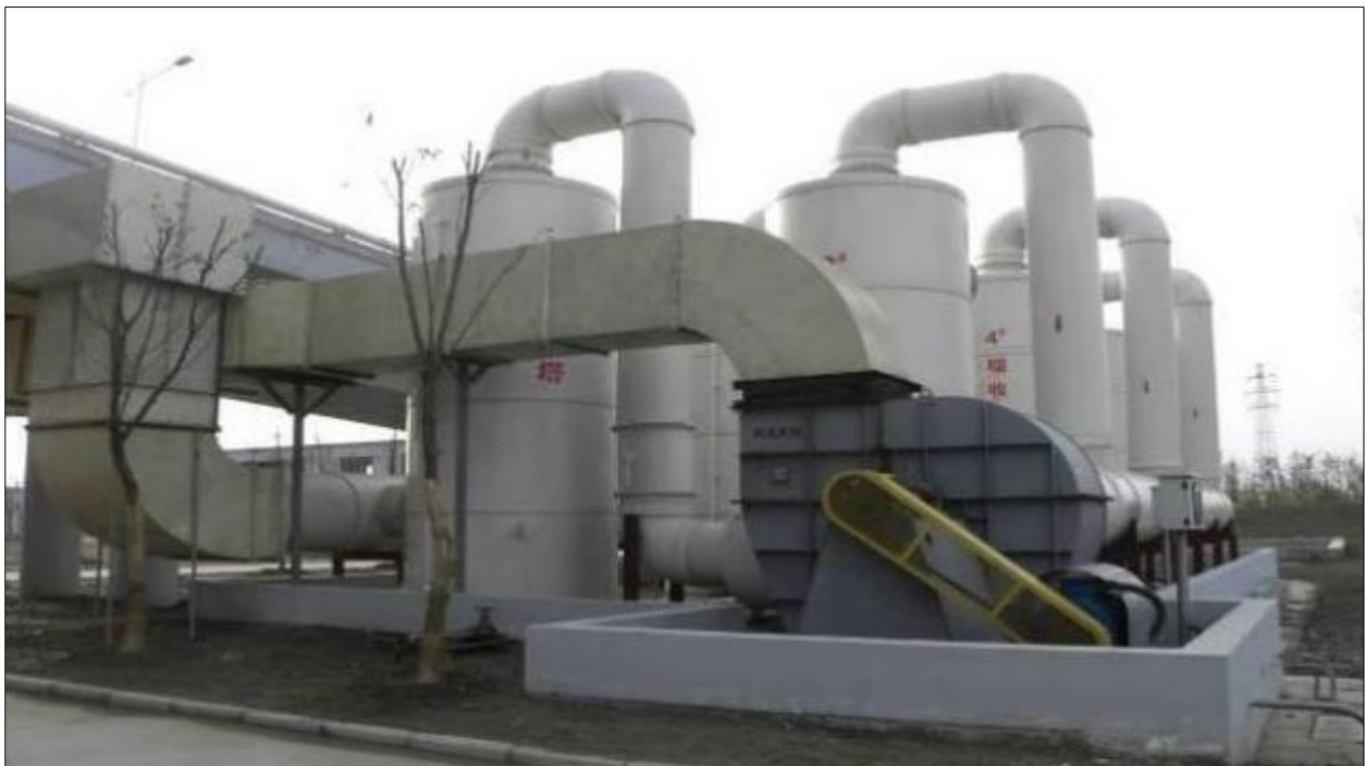
Figure 11: Waste Bunker Secondary Deodorising system showing extract fan and scrubbing towers.
