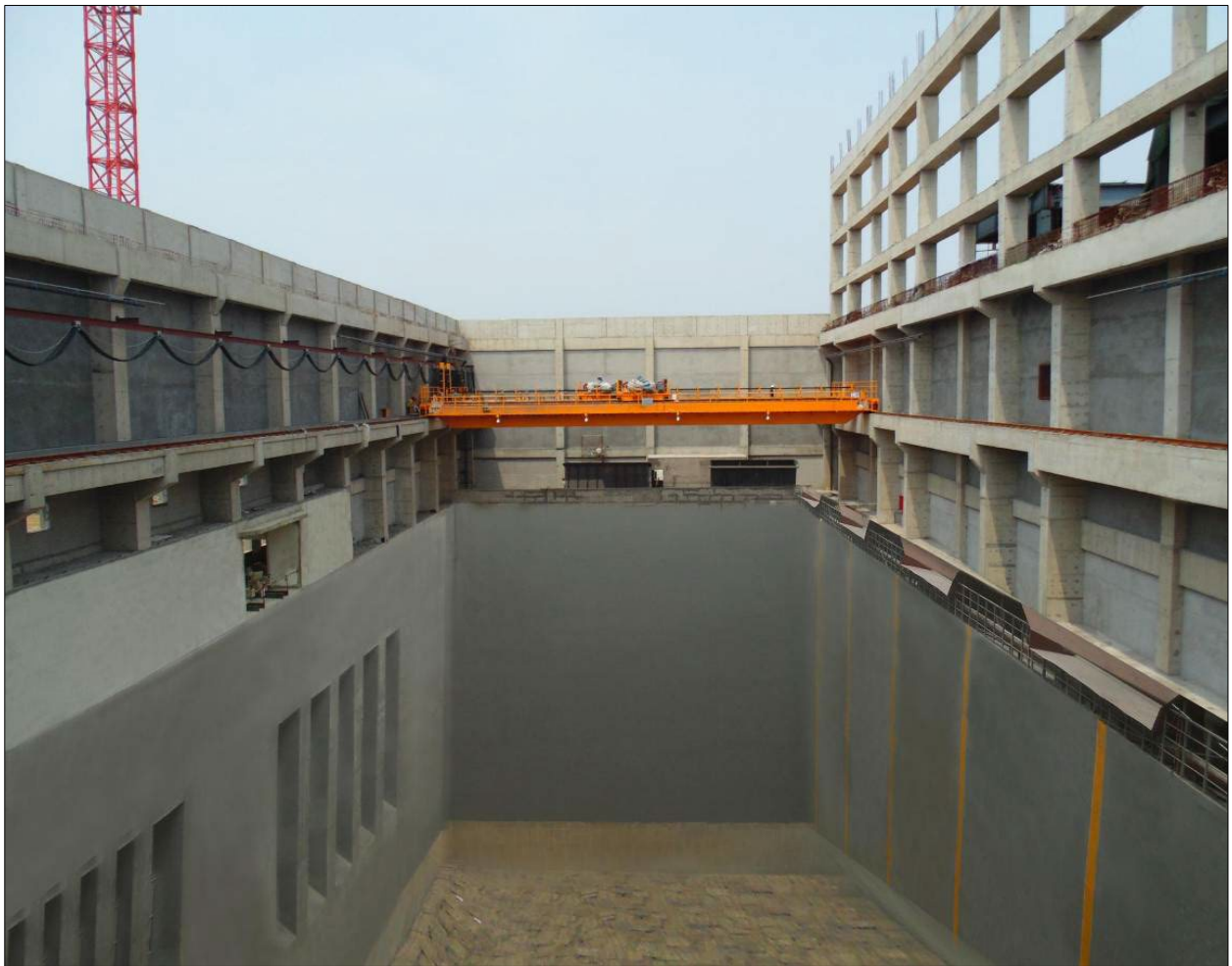
Figure 9: Waste bunker during construction with the gantry for the grapple hook installed.
