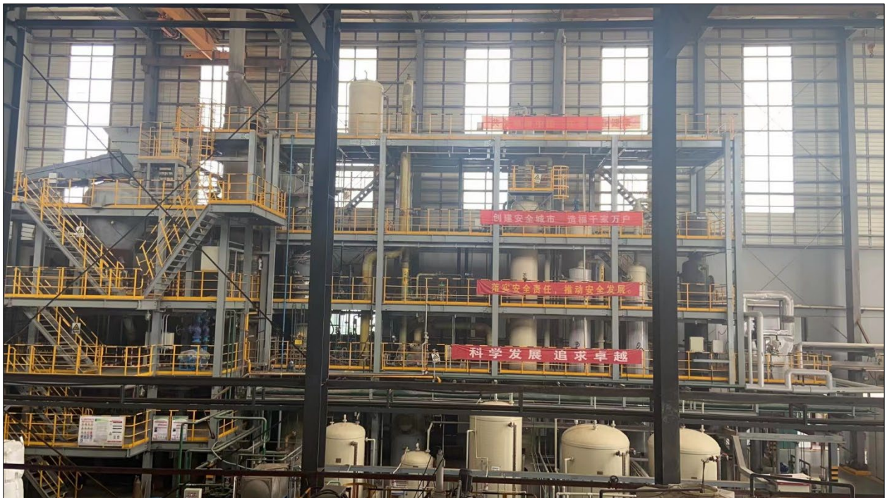
Figure 36: Plasma furnace (top left) and flue gas treatment process to the right
