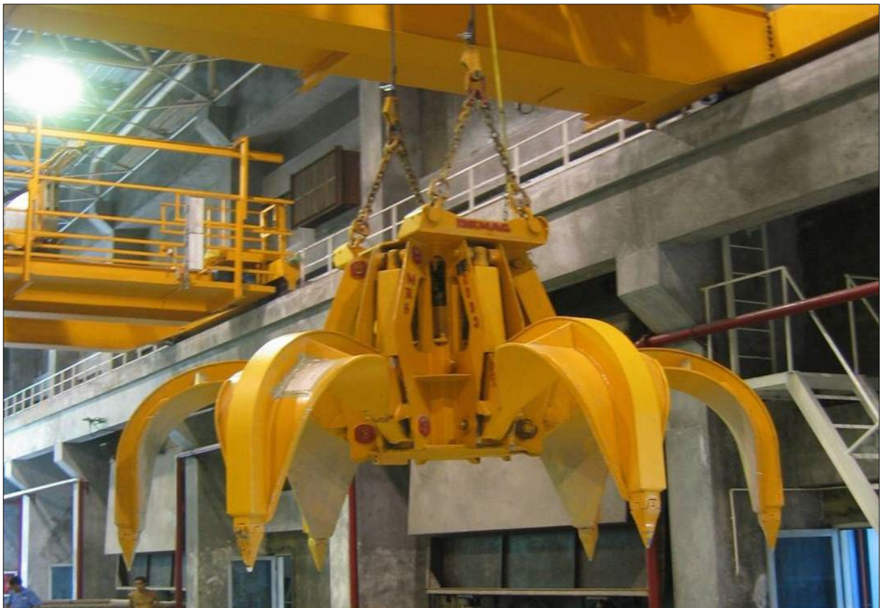
Figure 12: Grapple crane used to both mix MSW within the bunker and feed MSW into the furnaces.
